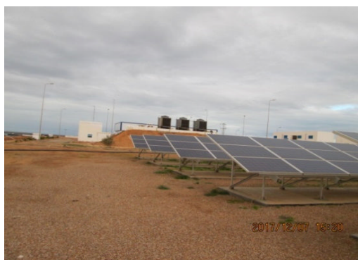
Photo 2: Solar Power Generation System
