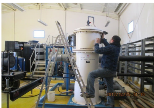
Photo1: Inside of Desalination Plant Facilities
