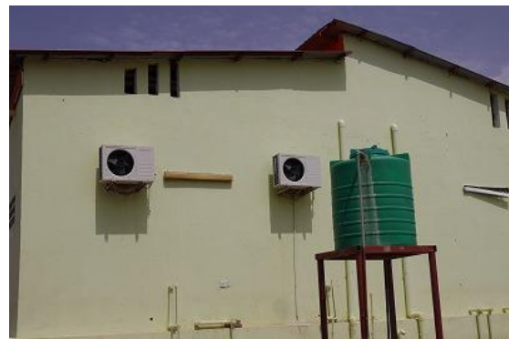
Rehabilitated Obstetric Care Unit at Suki Locality Hospital at the Time of Ex-post Evaluation
