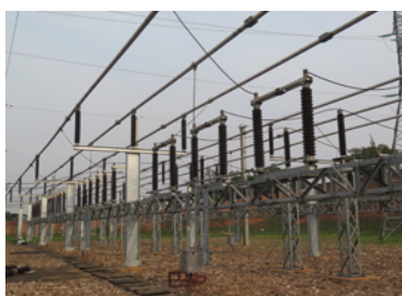
Outdoor switchgear (Gikondo Substation)
