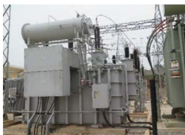
Main Transformer (Musha Substation)
