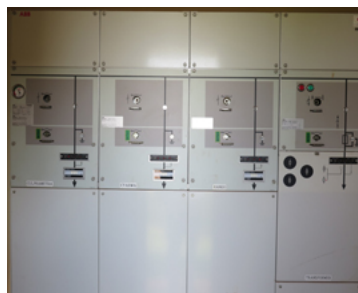
Ring Main Unit (Huye distribution network)
