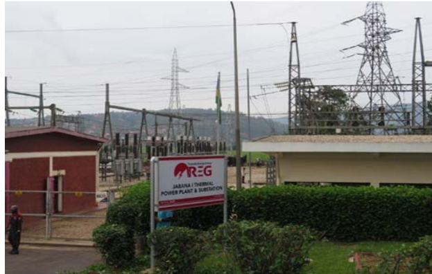
Jabana Substation Refurbished by this project
