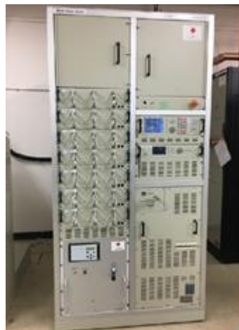
Short-wave transmitter (Henderson Transmitter site)
