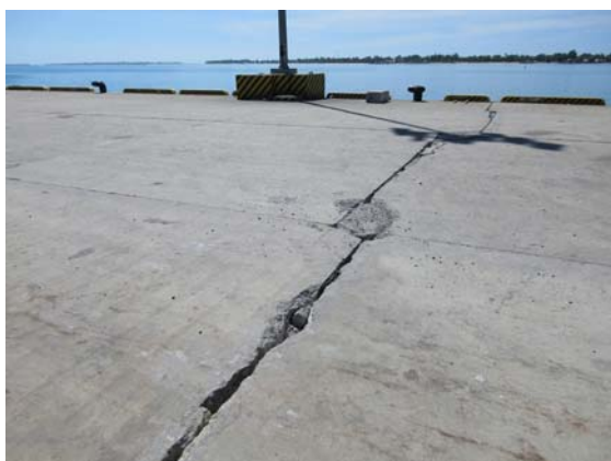
Damages to the Upper Surface of the Wharf
