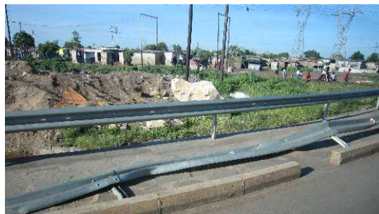
Photo: Damaged guardrails
