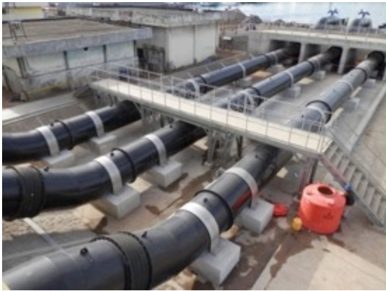
Photo 3: Pluit Pump Station Aboveground pipe line system
