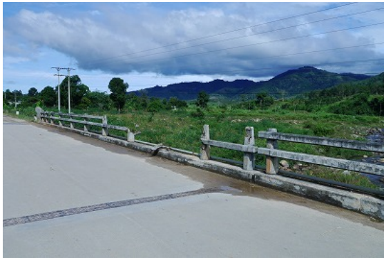
Ngoc Tu Bridge with broken guardrails by the severe flood in 2009
