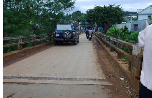
Ia Drang Bridge where drainage ditch is filled with dirt
