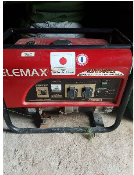
Generator in Savanakheth Office
