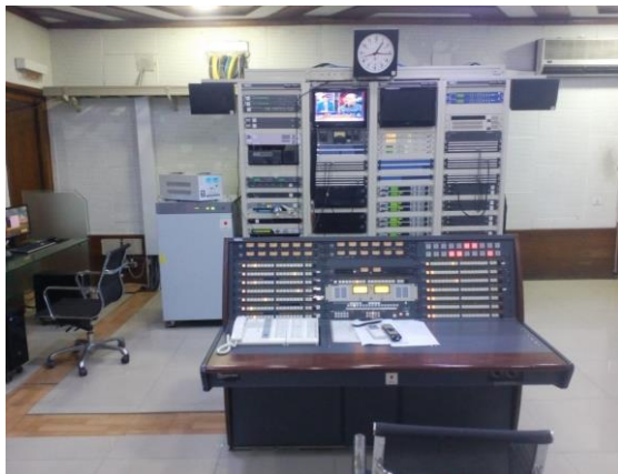
Master control room at the headquarters, Islamabad
