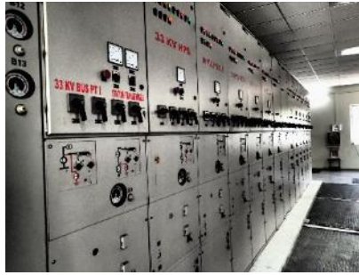
Control panel (Balkampet substation)
