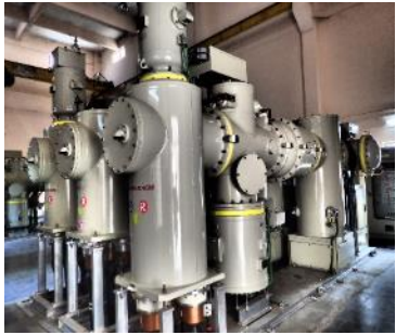
GIS unit (Patigadda substation)
