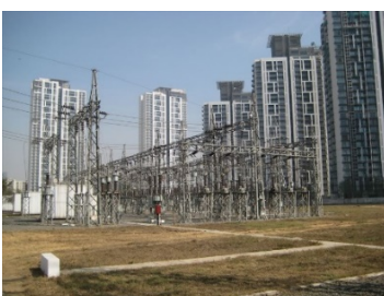
Sector 72 Substation (Gurgaon)
