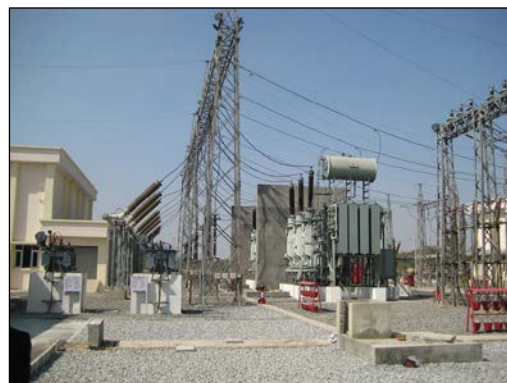
Sector 20 Substation (Gurgaon)
