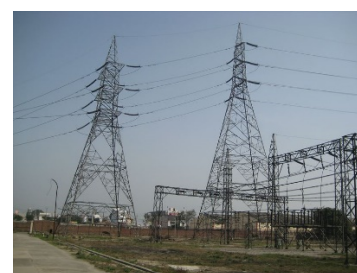
Power Line (Samalhka Substation)
