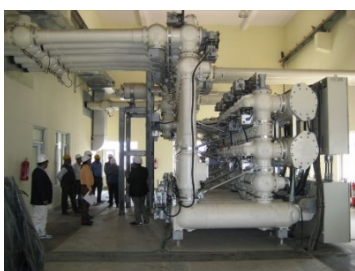
Sector 20 Substation (Gurgaon) Gas Insulated Switchgear (GIS)
