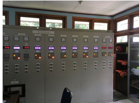
Photo 2: Water Gate Control Room of Babat Barrage
