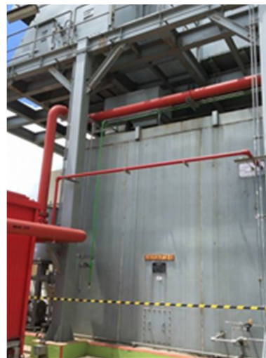
Photo 2: Generator for Gas Turbine Unit 1
