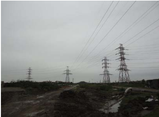
Ben Rung-Bac Song Cam Transmission Line (Hai Phong City)
