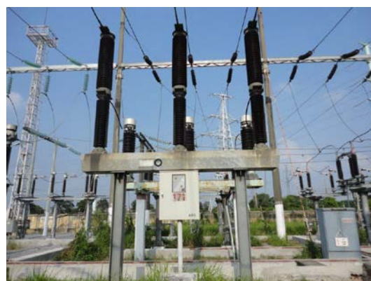
Quang Minh Substation (Hanoi City)
