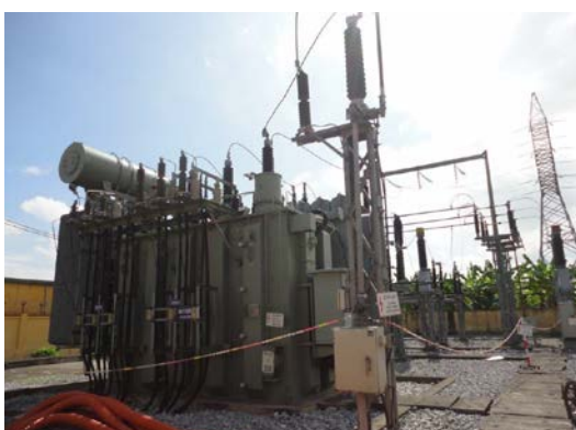
Chau Son Substation (Ha Nam Province)
