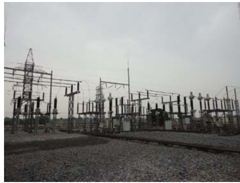
Yen My Substation (Hung Yen Province)
