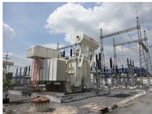
An Phuoc Substation (Dong Nai Province)
