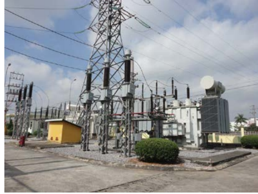
Phuc Dien Substation (Hai Duong Province)
