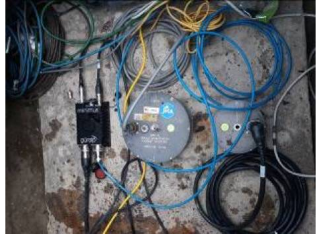
Accelerometers were all under operational and maintained properly by TDMMO
