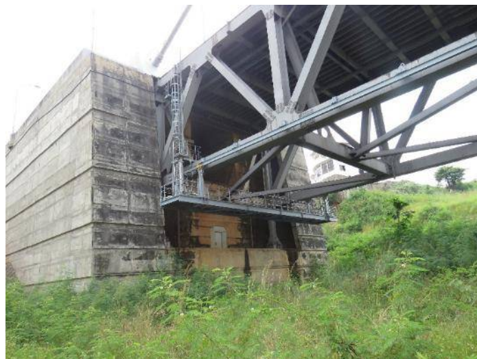
Inspection trolley (TC)
