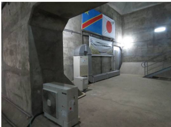
Injection dry air system machine (GA)
