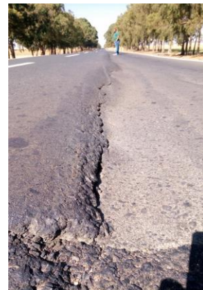
Settlement of the road surface partly due to influence of black cotton soil
