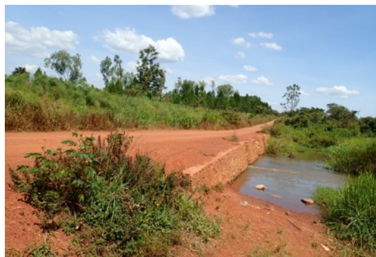
Photo 2: Access road and river crossing and road-drainage culvert developed by this project
