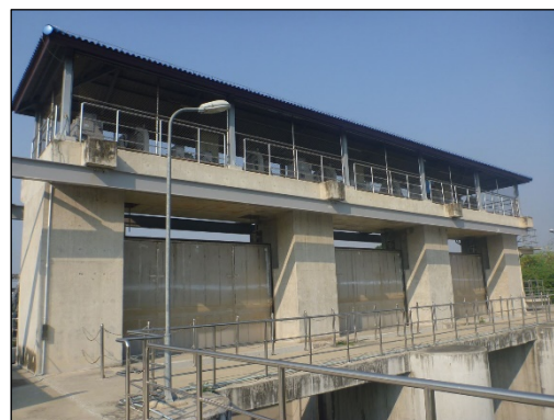
Photo 3: Kra Mang Floodgate
