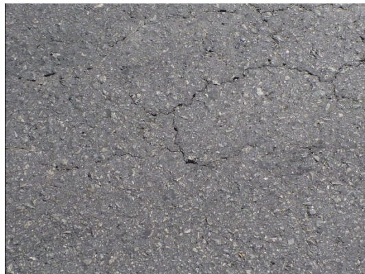
Photo 3: Cracks on the Pavement
