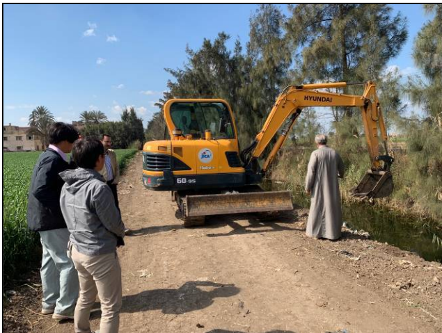
Excavator procured by the project is used for regular cleaning of canals in Bisintaway, under the observation of the Chairman of the BCWUA.
