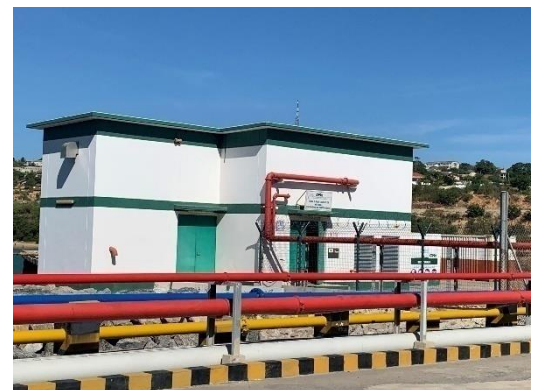
Firefighting system (Pump facility)
