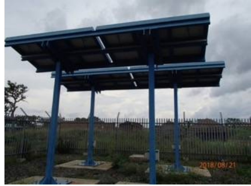
Solar Panels installed in Corner Kilak (the power systems inspected seemed to be in good condition)
