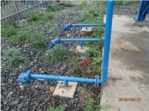
Distribution pipes in Corner Kilak are intact
