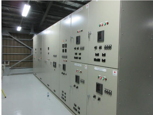
11kV high voltage receiving panel (at the Vaini project site)
