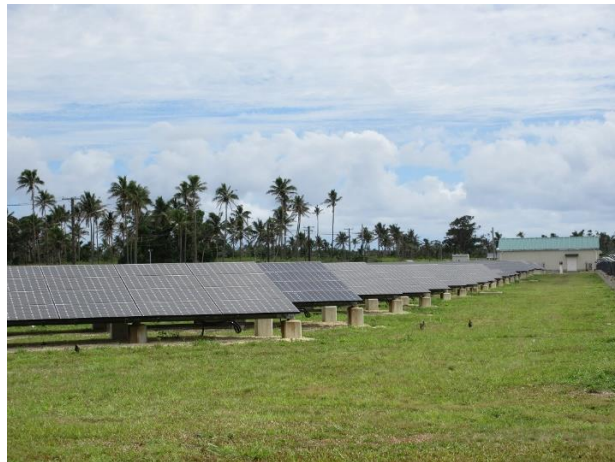
Solar panels installed in this project
