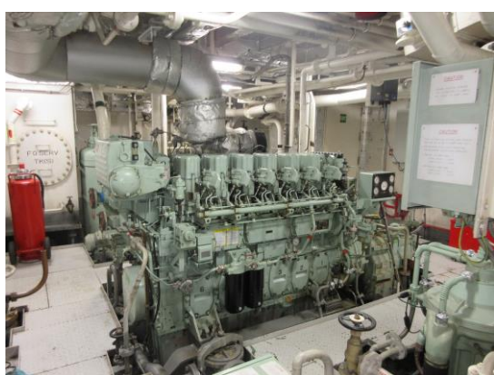
Inside the engine room
