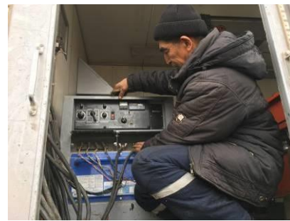
Inside of the mobile workshop van
