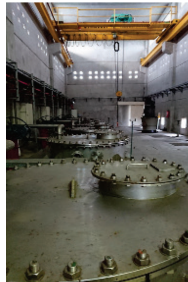
Pumps of the Semarang Pumping Station
