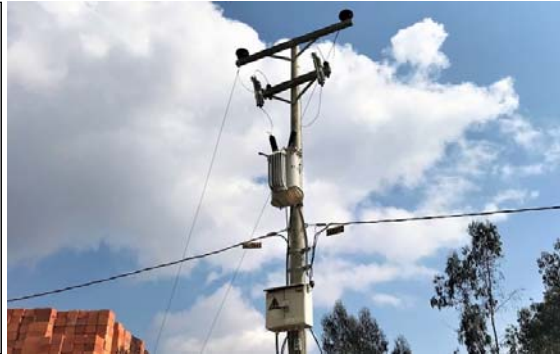
Distribution facilities provided by the Project
