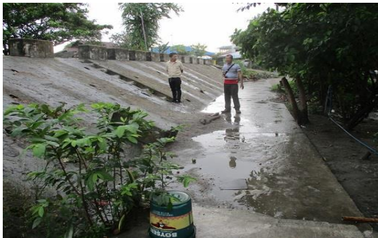
The old road (Center in the photo) and the new road raised by the project (Upper left in the photo)
