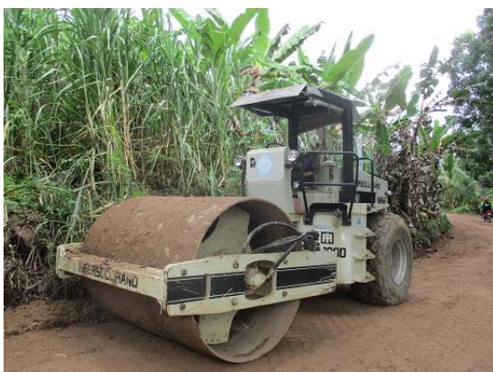
Maintenance of unpaved agricultural roads using heavy equipment purchased through a sub-loan project (Municipality of Ayungong)
