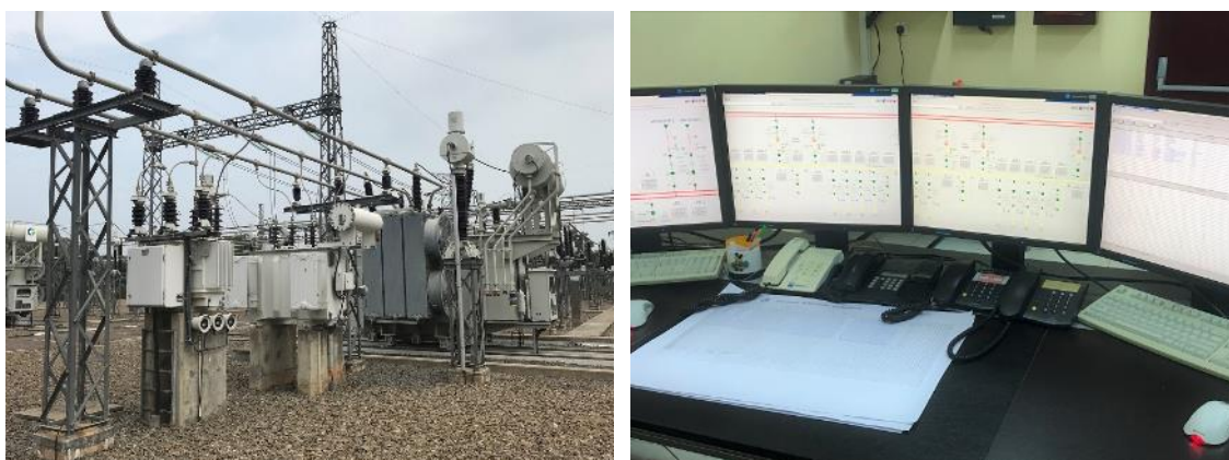
Kilinochchi Grid Substation: (left) Transformer facilities, (right) Monitoring panel
