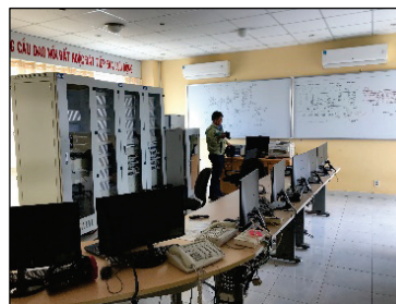
Photo 7: My Tho 500kV Substation Operator Room
