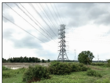
Photo 2: 220kV Duyen Hai – Tra Vinh Transmission
