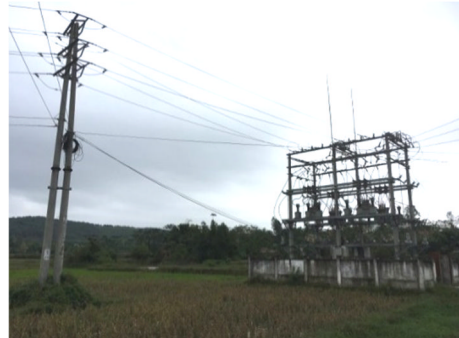
Picture 4: Developed Distribution Networks and Transformers
