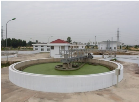
Picture 3: Developed Waste Water Treatment Plant (Vinh Yen Waste Water Treatment Plant)
