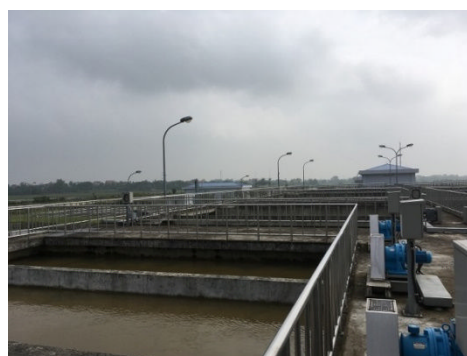
Picture 2: Developed Water Treatment Plant (Vinh Yen Water Treatment Plant)
