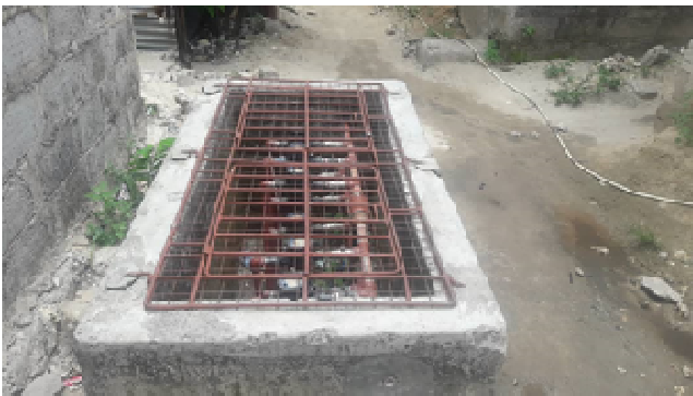
Manifold showing the water meters installed for house connection for ten households introduced by the phase 2 project (At Makadara area)
