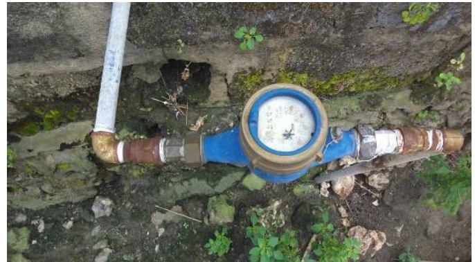
The water meter connected to single household; old style used by the phase 1 project (At Makadara area)
