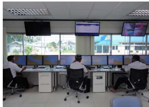
Operation Room at Dumai VTS Center
