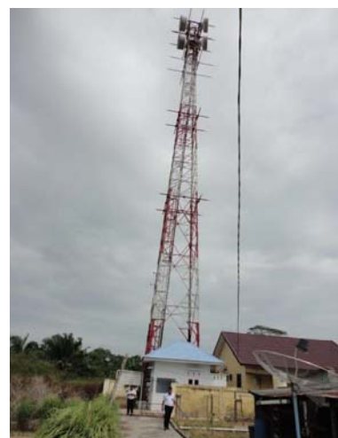
Exterior of Selincing Repeater Station
