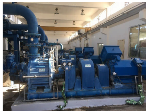
Pumping Station Developed by This Project (Zarqa Pumping Station)
