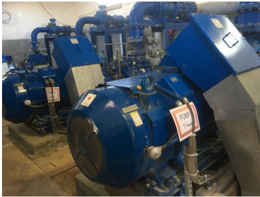
Photo 1: Pumping Facility at Hallabat Pumping Station
