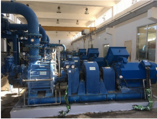
Photo 3: Pumping Facility at Zarqa Pumping Station
