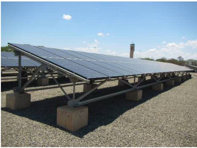
PV modules (the solar panels)
