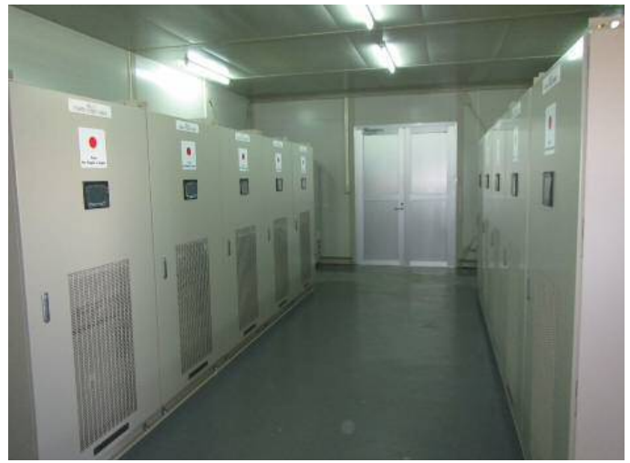
Power conditioners in the energy conversion room
