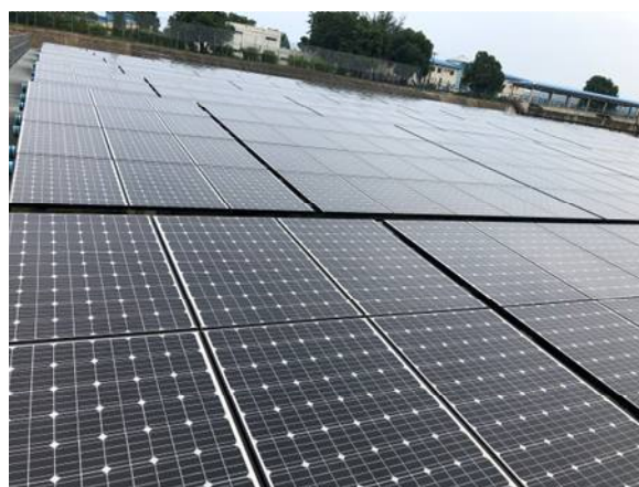
PV modules installed under the project
