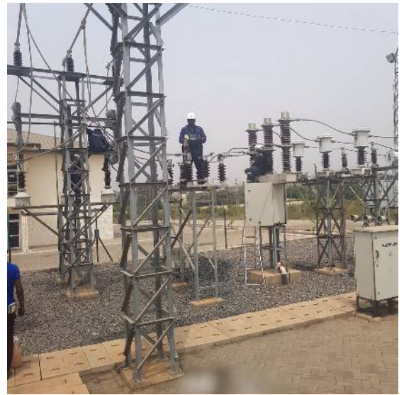
Training course for ECG Technicians on Sub-station maintenance
