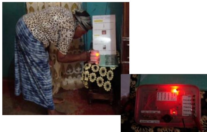
WRUA explaining operations of functioning Early Warning System equipment in Upper Lumi (Left). Properly functioning Early Warning System equipment in Upper Lumi (Right).
