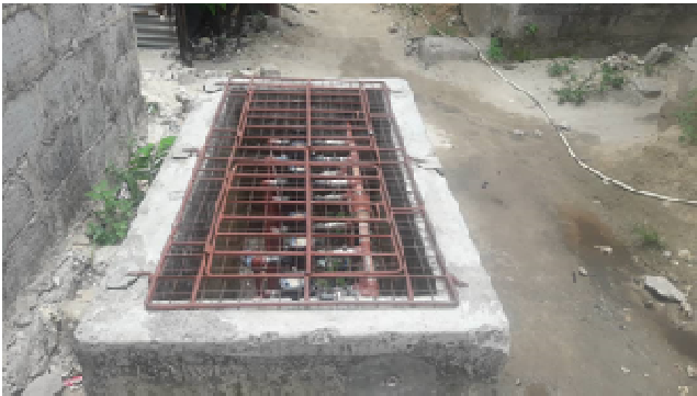
Manifold showing the water meters installed for house connection for ten households introduced by the phase 2 project (At Makadara area)
