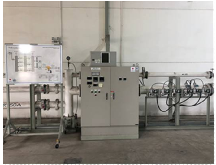
The training facility at Energy Management Training Center in HCMC
