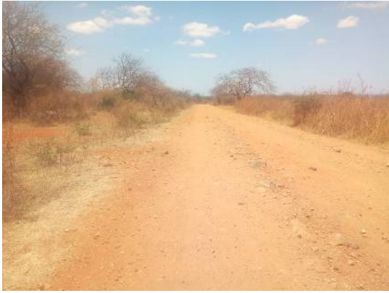
Nkwenda - Nhinhi road in Dodoma Region one of the pilot projects of the project
