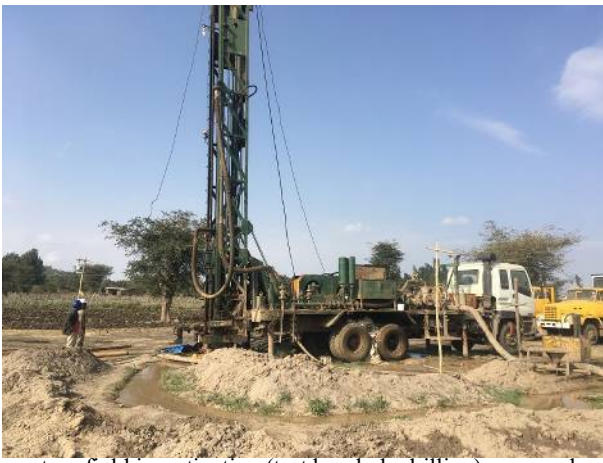
Preparatory field investigation (test borehole drilling) proposed and implemented as a result of this project
