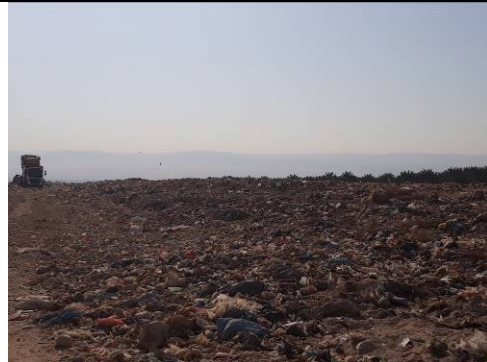
The expansion of Jericho Landfill, implemented by UNDP, enabled Jericho JSC to sustain their SWM services
