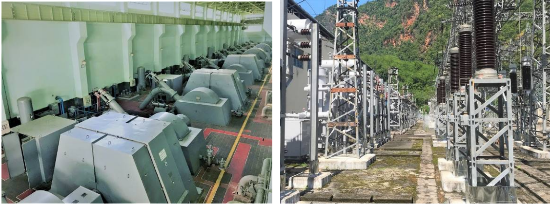
Baluchaung No.2 Hydropower Plant: generating equipment (left), substation equipment (right)
