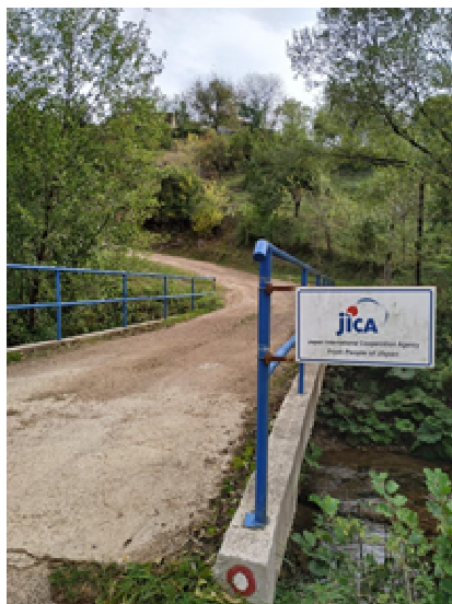
Bridge in Zlicina Village, Constructed under the Project, Promoted Rural Tourism Development (Rogatica Municipality)
