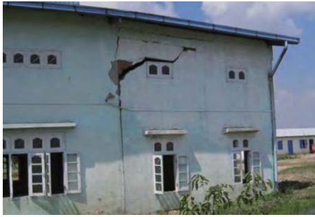
Pump House (at the time of planning)
