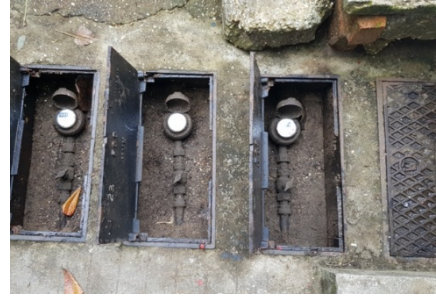
Individual water meters installed in Yankin Township
