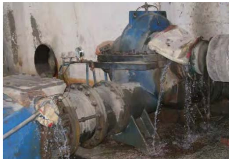
Transmission and Distribution Pump (at the time of planning)
