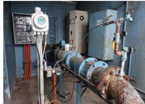
Well Pump Station Electro-Magnetic Flow Meter, PLC Board
