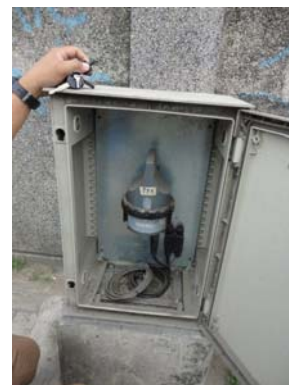
Pressure Sensor at Water Pressure Monitoring Point
