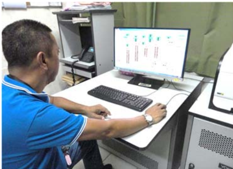
SCADA Client in Talamban Satellite Office
