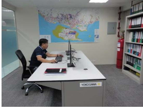
SCADA Room inside the MCWD Main Office
